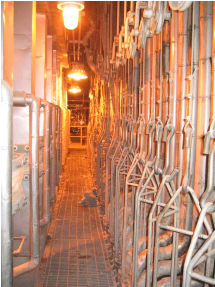
Pre Incident General Radiant Tube External Arrangement
