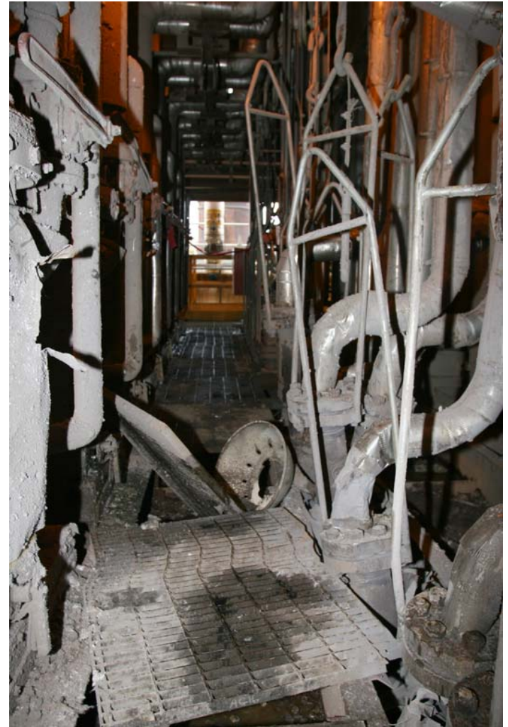
Post Incident External Damage
